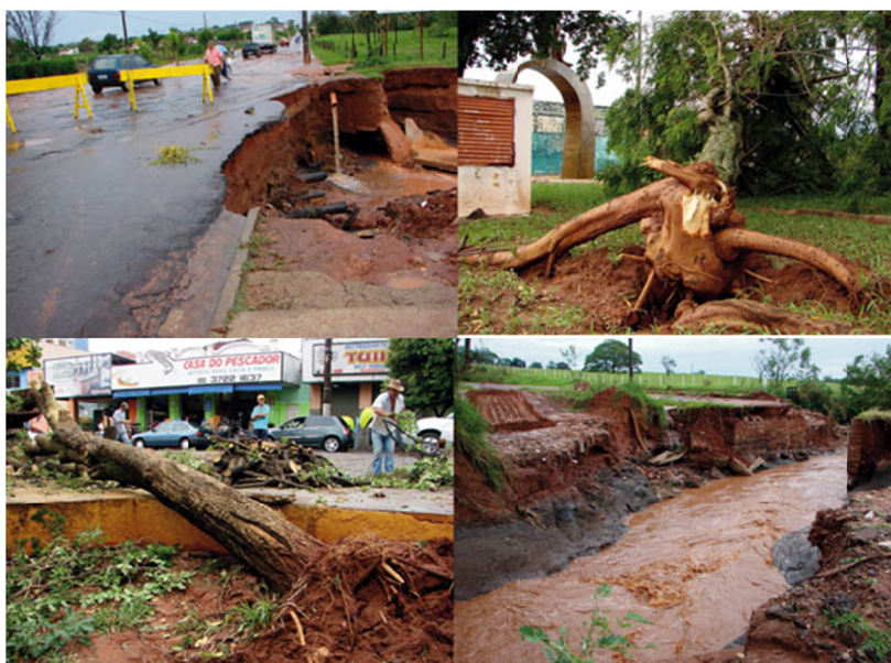
Figure 9. Damage caused by the extreme event of 15 October 2009 in Andradina (Source: journal Jornal Regional edition of 16 October 2009)
